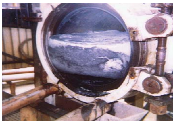
Figure 1—Gas hydrates plugs (Crumpton 2018).
